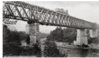
Seneca Ray Stoddard Adirondack R.R. Bridge across from Sacondaga Gelatin Silver Print
